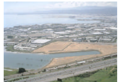
Bay West Cove (1998) The site after onshore remediation and ready for development. Highway 101 is in the foreground and the Oyster Point industrial/office park (including Genentech) is in the background.
